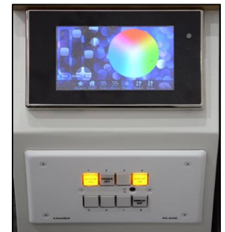
Touch panels to remotely power-up amp racks, console and for room lighting
